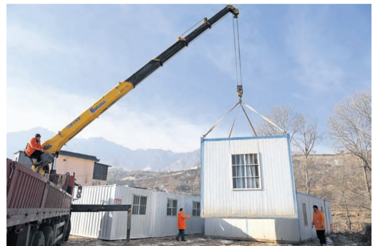
In this photo released by Xinhua News Agency, movable plank houses for earthquake victims are set up in Meipo Village, Jishishan County in northwest China's Gansu Province, Thursday, Dec. 21, 2023.
